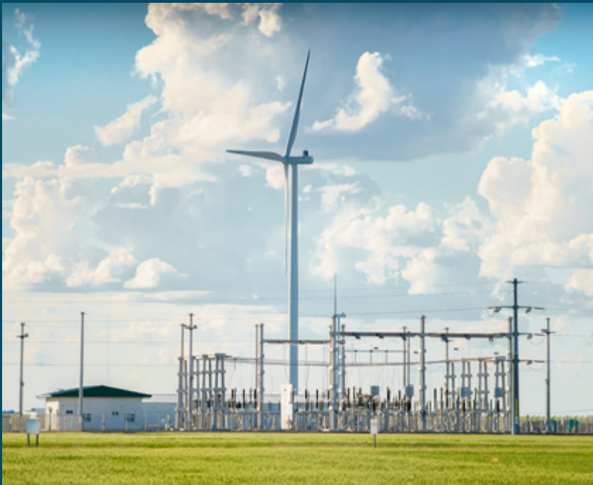
Windmill Power Generator and Transformer Station
