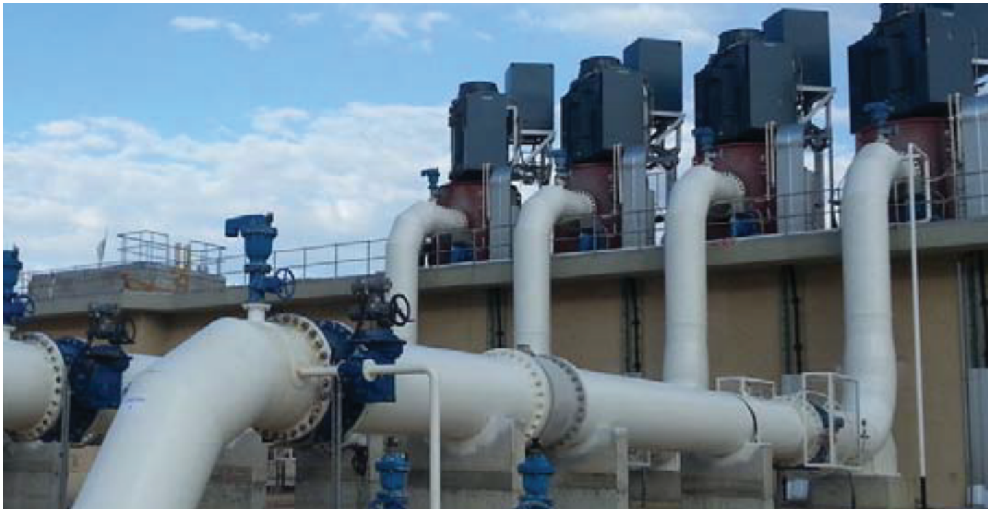
Water pump station at Mekorot Israel
