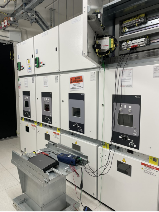
Power Quality Analyzer installed in medium voltage side (upstream B2_MV/LV_Tx)
