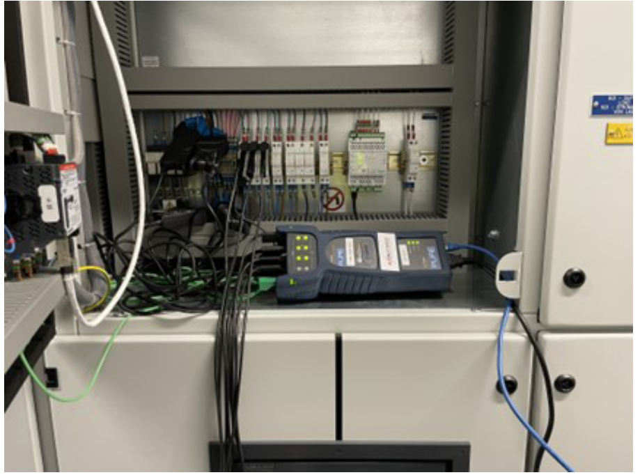
Power Quality Analyzer installed in low voltage side (upstream B1_UPS)
