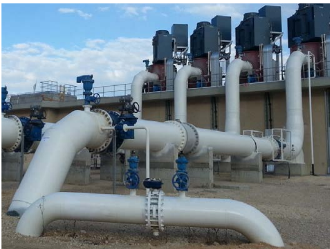
Water pump station at Mekorot Israel
